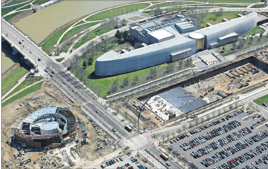
A quick spin through Downtown and the Ohio State University area reveals there is a lot of construction going on around town. Here, work continues at the National Veterans Memorial & Museum site on the left — the former site of Veterans Memorial — and on an underground parking garage next to COSI. The Scioto River is at the top. [CRAIG HOLMAN /DISPATCH, ABOARD WBNS CHOPPER 10]
